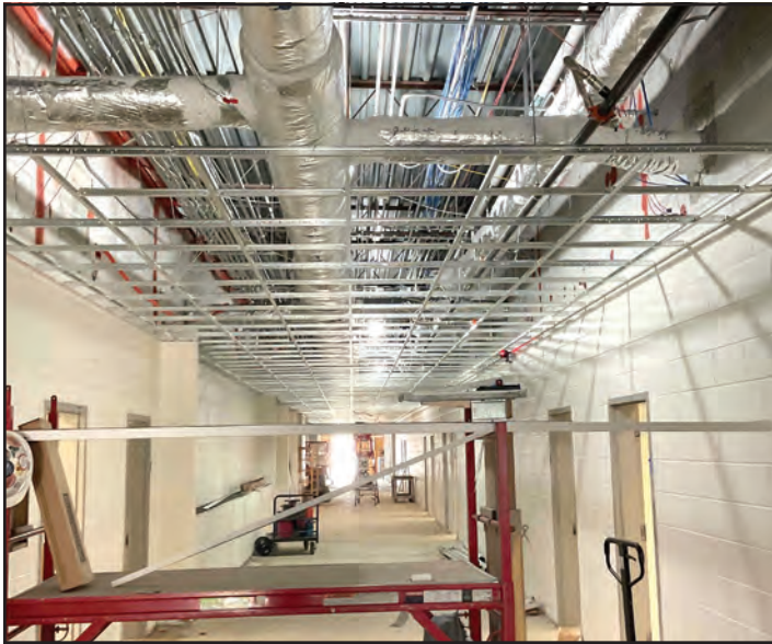
'D' hall renovations are in full swing and are planned to be completed by June 6.
