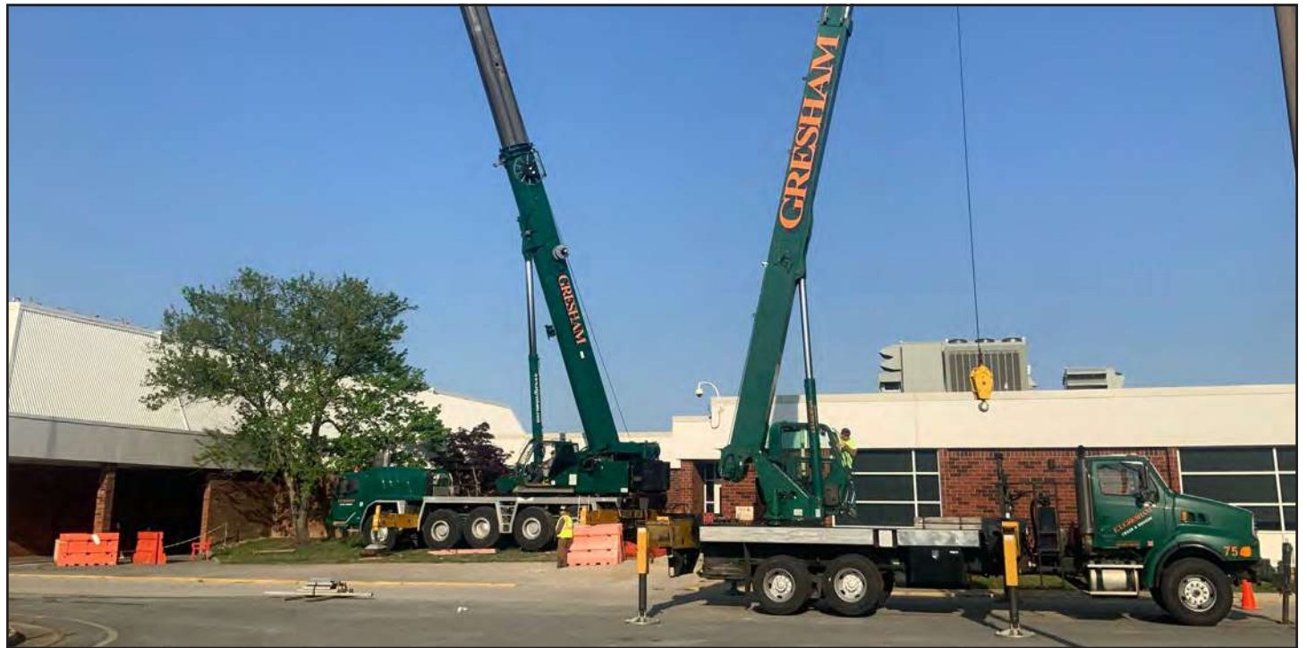
Gloucester High School will have new HVAC units installed as part of the renovation process. Pictured are old HVAC units being removed from the school.
